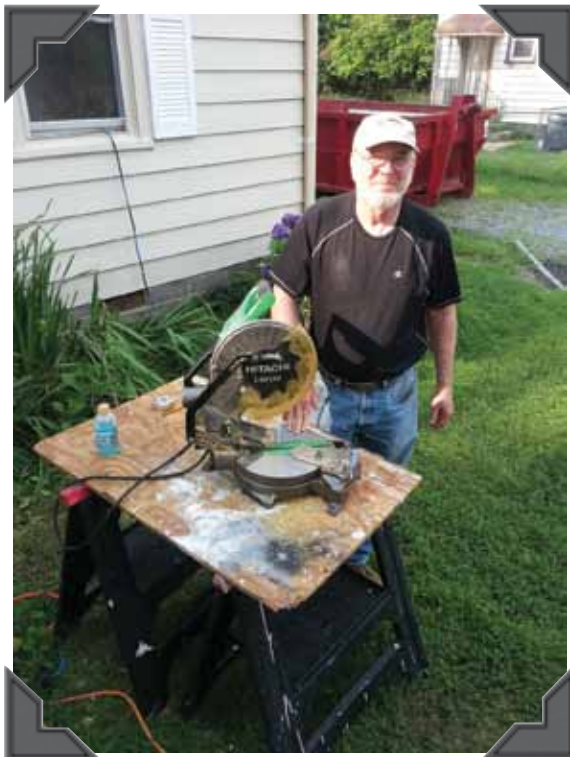
Ken Hoen was on the Richmond Outreach Ministry team working construction in the East End.
